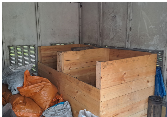
New coal bunkers
